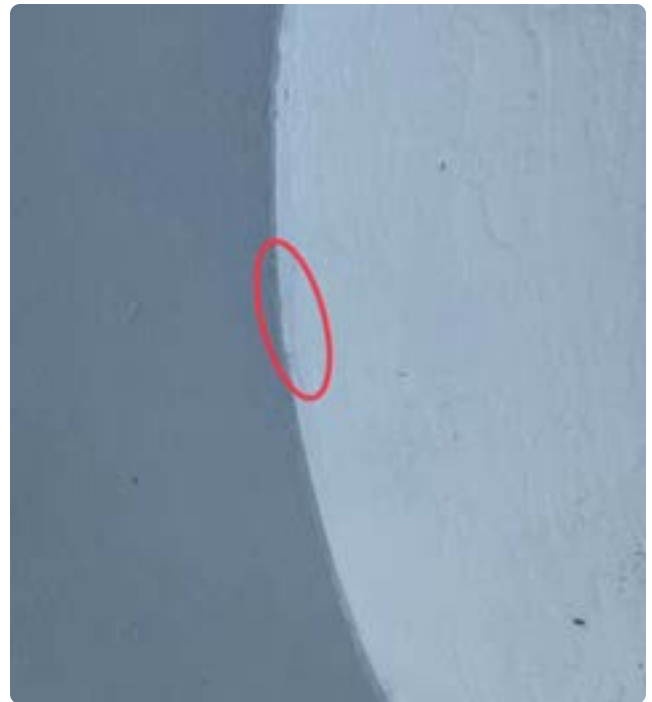
Cracking at walkway to wall connection outside unit 6059
