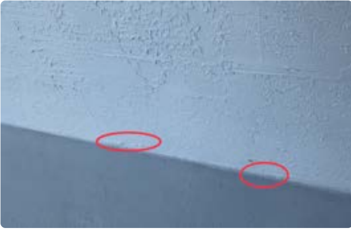
Cracking at walkway to wall connection outside unit 6023
