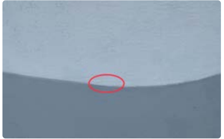
Cracking at walkway to wall connection outside unit 6021
