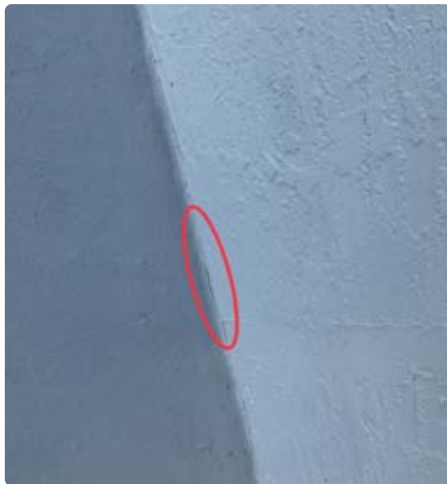
Cracking at walkway to wall connection outside unit 6023
