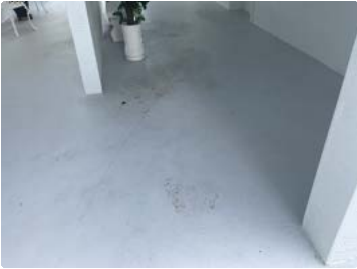
Delamination on first floor walkway
