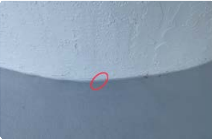
Cracking at walkway to wall connection outside unit 6037
