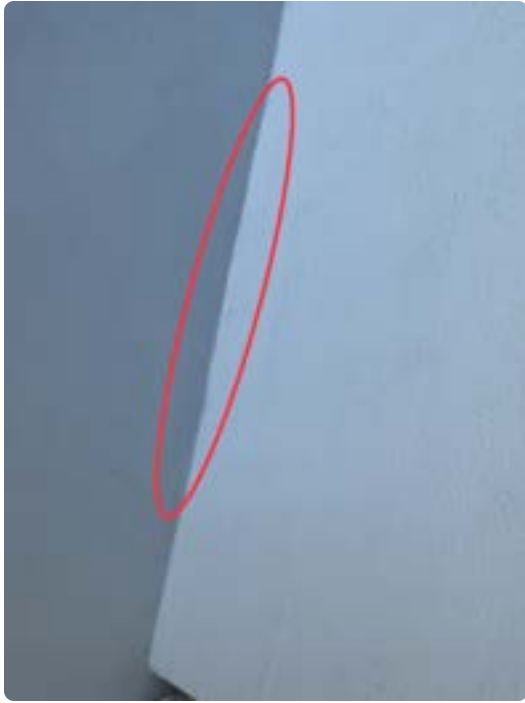
Cracking at walkway to wall connection outside unit 6055
