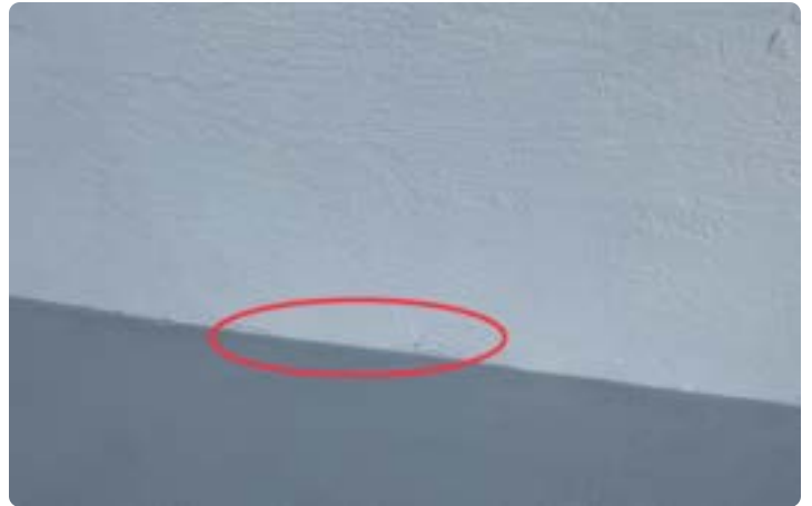
Cracking at walkway to wall connection outside unit 6041
