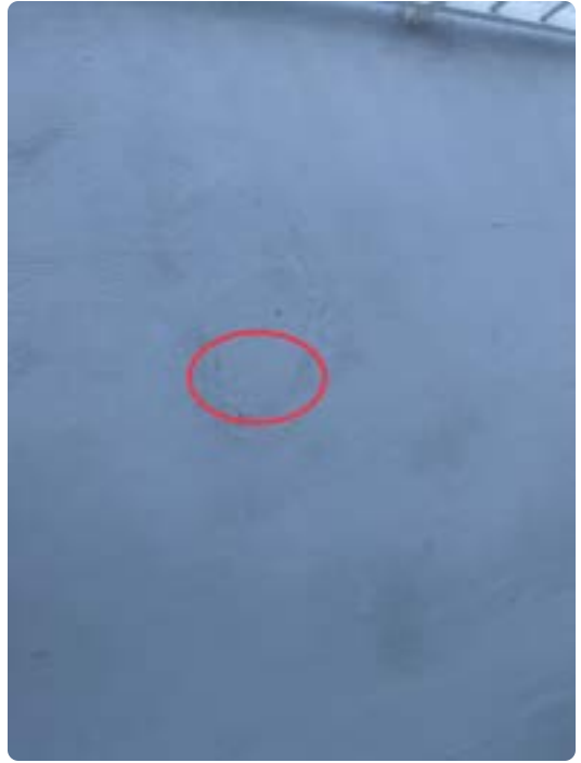
Debanded coating outside unit 6027
