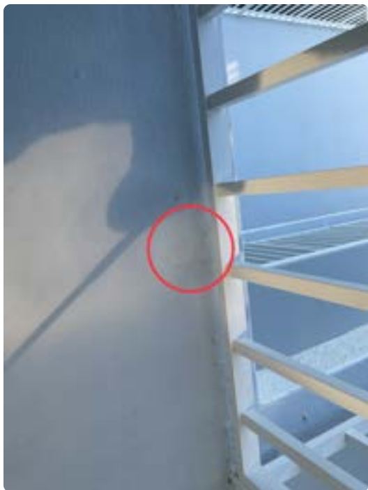
Debonded coating on walkway outside unit 6039
