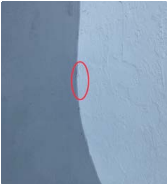
Cracking at walkway to wall connection outside unit 6045
